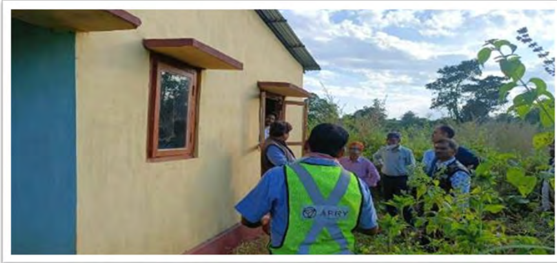
ADB's Social Safeguard Expert and CGM (PP&I) visited the relocation site under development and sample model house constructed
